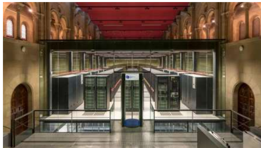
Marenostrum IV Barcelona Supercomputing Center
